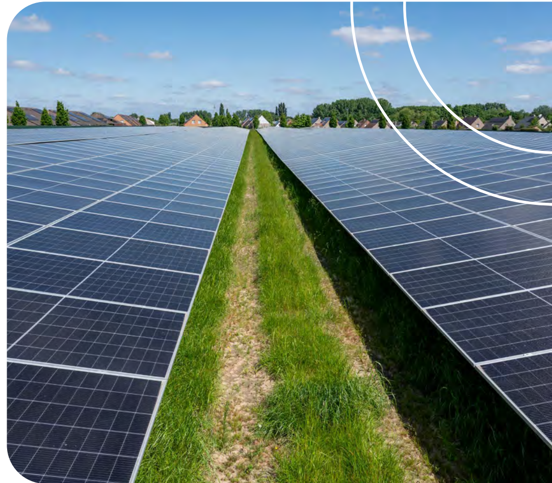
First solar park, built on land owned by a social housing company in Lauwe. Nearly 8,000 solar panels will provide 400 households with green electricity each year.
