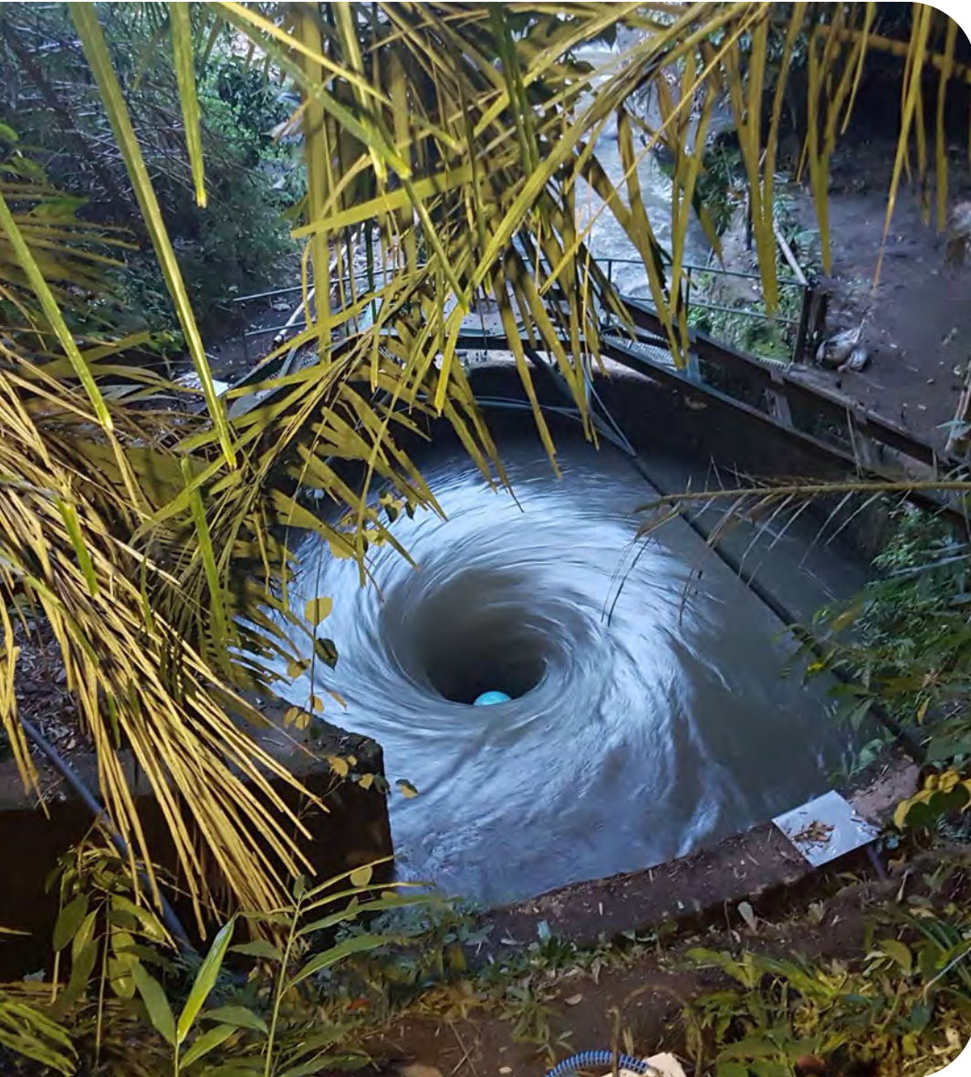
A Turbulent installation in Bali, Indonesia.
